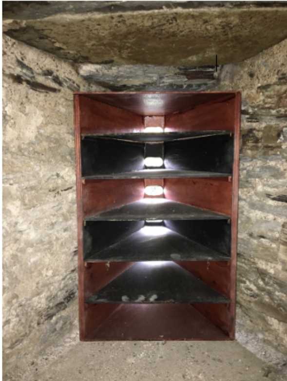
Boxes installed at Bere Ferrers church in an arrow slit as there is not enough space in the belfry.
