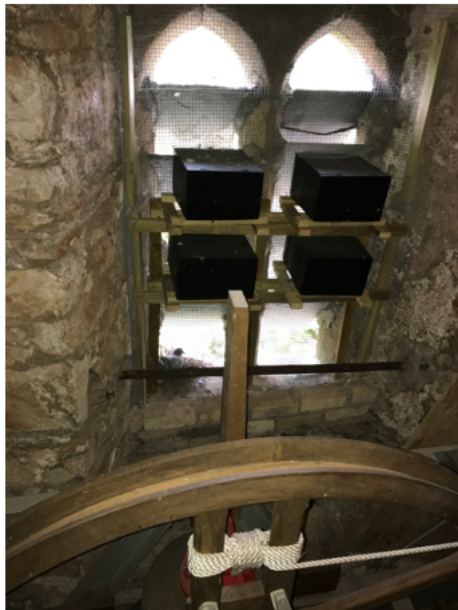
4 double decker boxes on a frame installed on the north aspect at Kingskerswell
